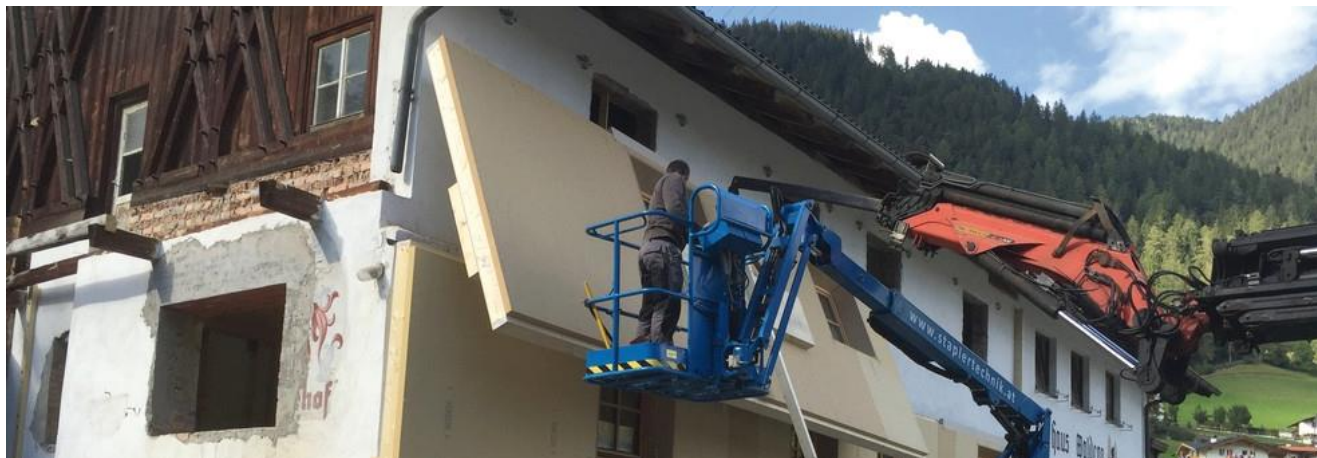
The 27 th International Passive House Conference will focus on exemplary building retrofits: the 300-year-old Mayerhof in Tyrol was equipped with prefabricated insulation made of wood fibre boards, Passive House principles . © Michael Flach
